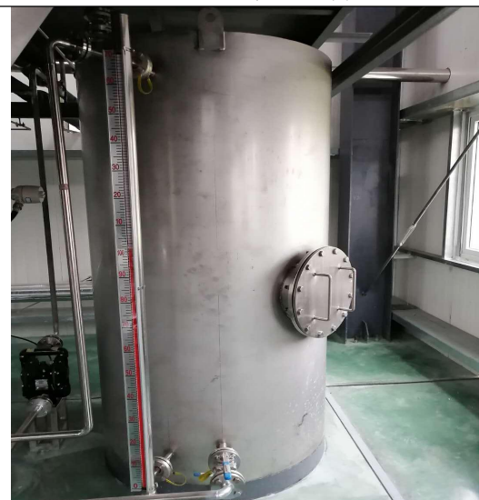
喷雾制粒正己烷回收罐
